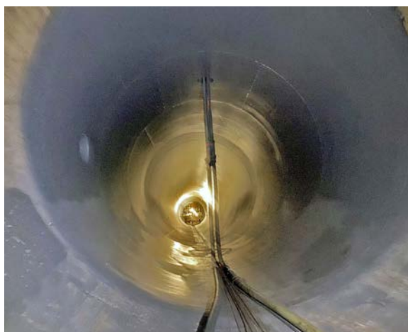
Grand Coulee Unit G8 penstock newly applied lining, from the concrete/steel transition to scroll case.
