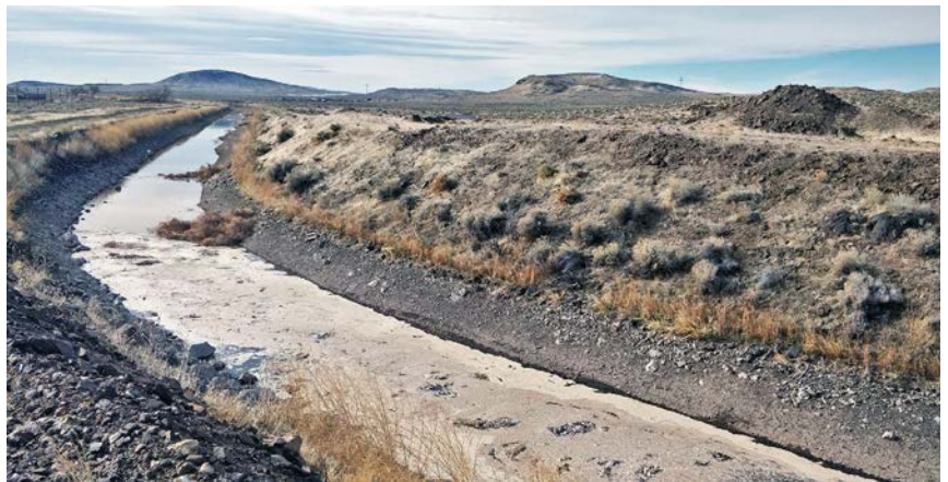
Unlined section of Truckee Canal from the heat-as-a-tracer seepage investigation. Photo credit David Smith, USGS.
